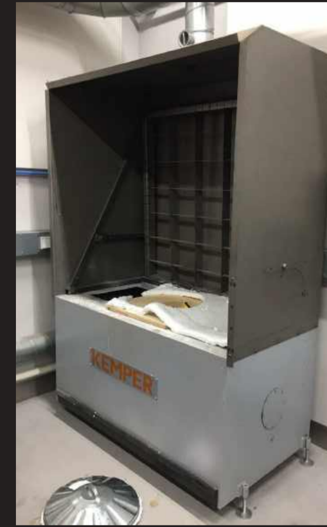
4-Extract fan is on and cut insulation.
